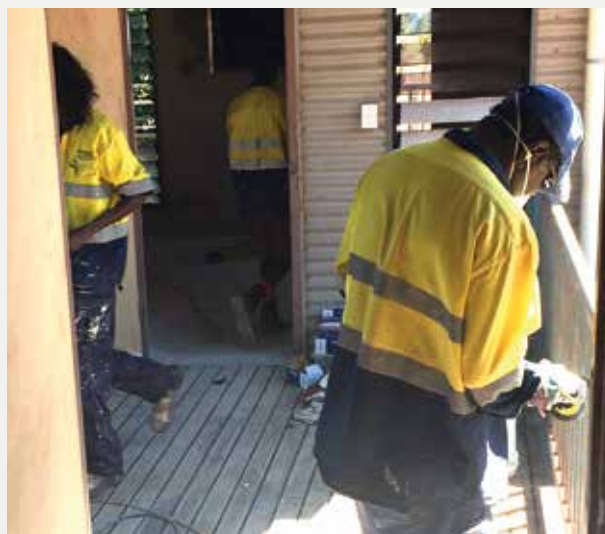
Galiwin'ku, DRG Industries local employees hard at work fixing one of the community houses damaged by Tropical Cyclone Lam in order to get the displaced family back in. Over 50% of the construction team that repaired the cyclone damaged houses in Galiwin'ku are local Yolngu.
